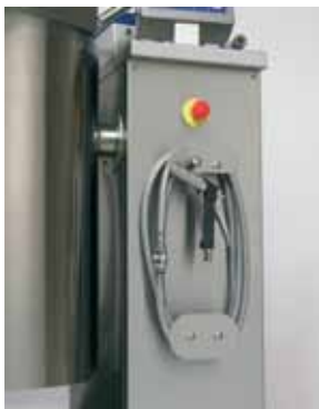
Hose reel mounted on the front of the pillar and hose connection on the top
